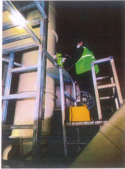
蚀刻工序废气处理后排放口 DA007
